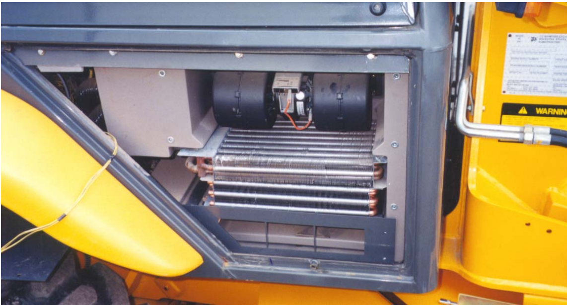
Evaporator in place beneath heater coil and blowers.
